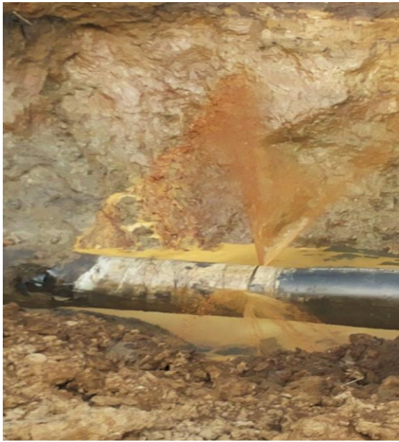
CRUDE OIL SPILLING OUT
